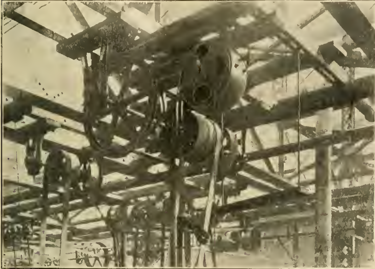
TYPICAL ARRANGEMENT OF CEILING MOTOR FOR GROUP DRIVING. LIGHT TOOL SECTION OF MACHINE SHOP.
